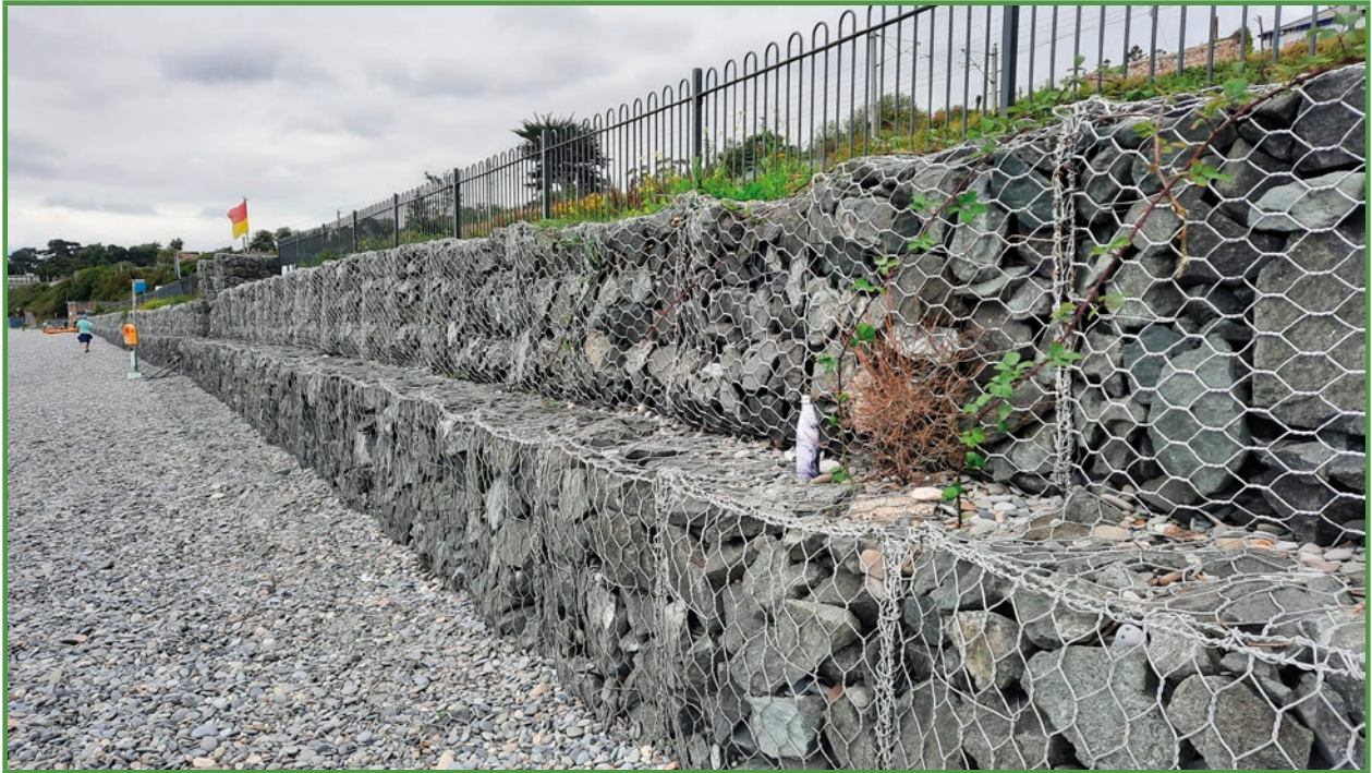
An example of a hard engineering solution is the installation of gabion baskets or cages which are used to protect the coastline against the erosive power of waves during storm events.
