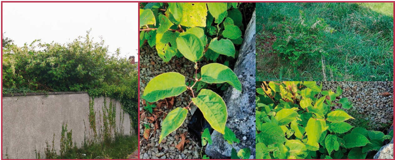
An infestation of Japanese Knotweed found adjacent to Athlone Train Station.
