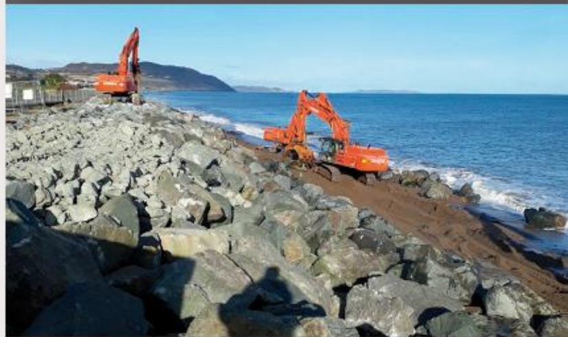
55t Excavators placing 10 ton boulders in to place at the 18mp Ballygannon
