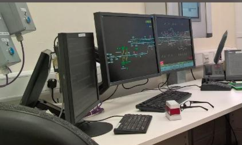
New Control Room at Limerick
