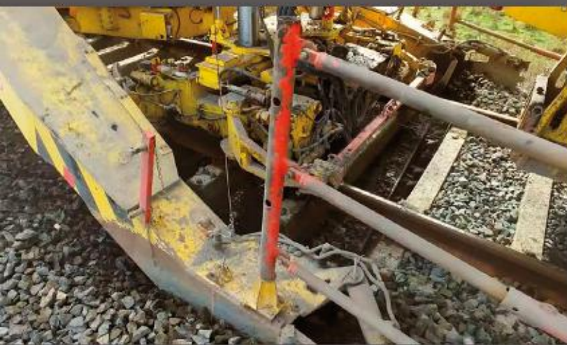
Figure 4 The Ballast Cleaner cutting bar removing the ballast from underneath the track
