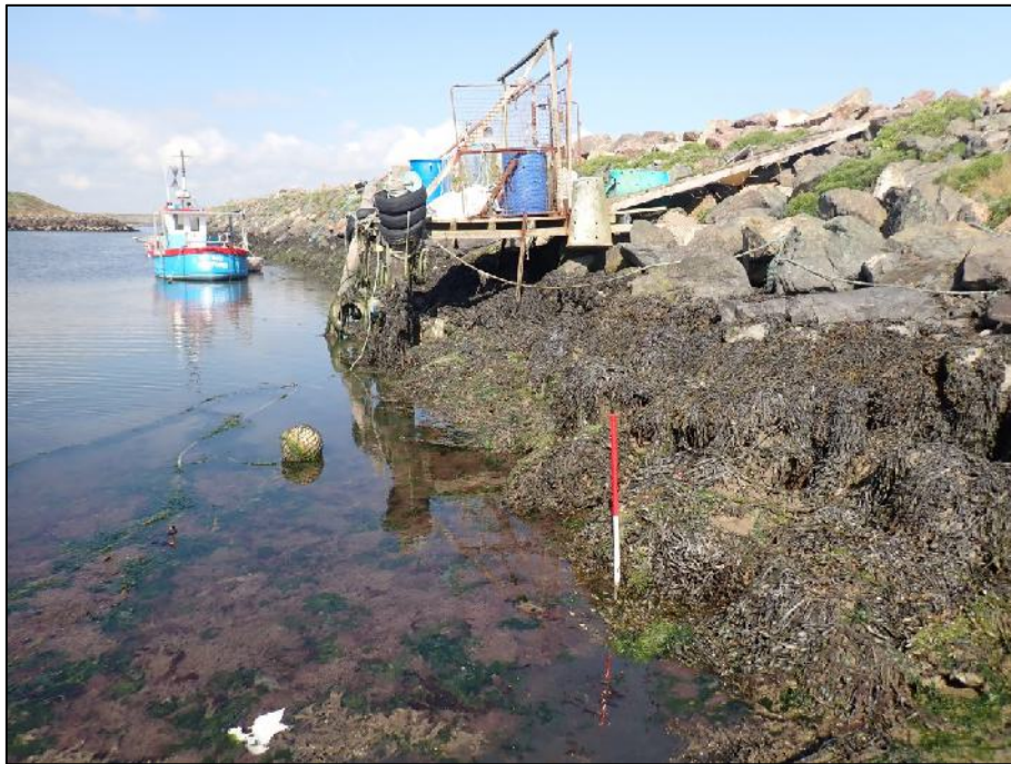
Plate 9: West-facing view of rock-armour revetment forming east side of the northern half (outer part) of the harbour area (1m scale).
