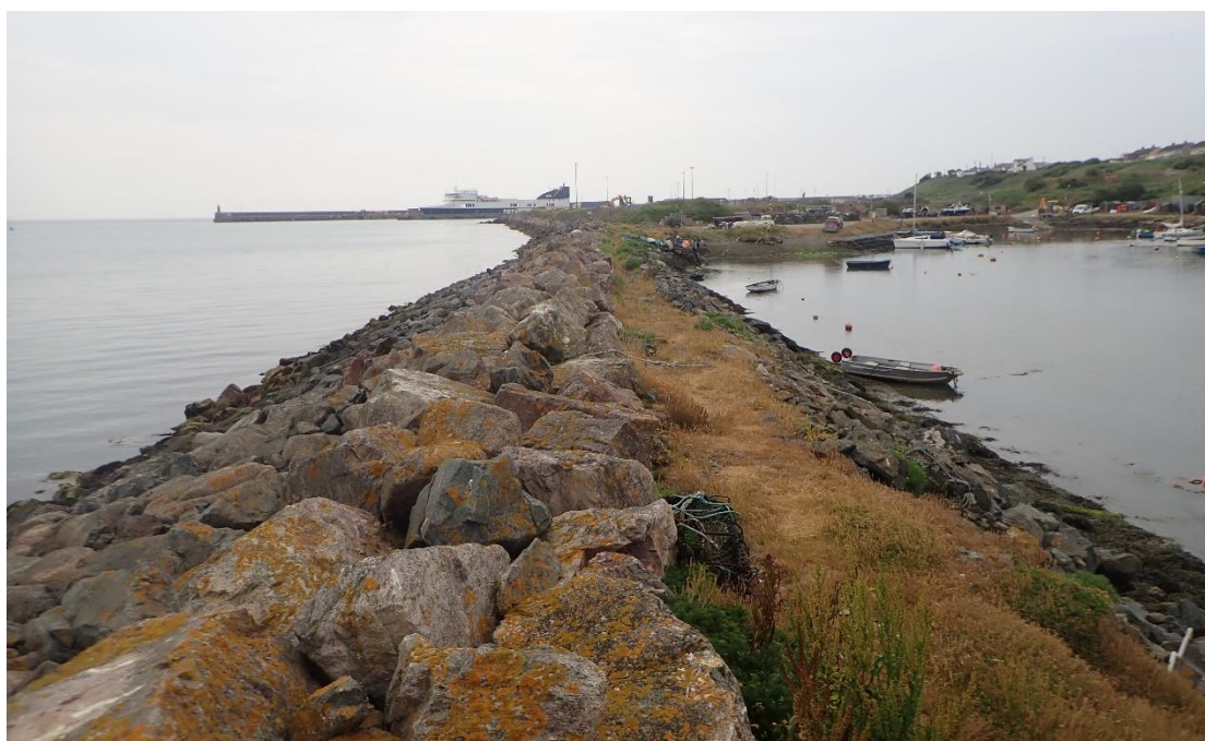
Plate 5: View looking east along northern breakwater in Ballygeary Harbour and across to the pier head in the distance.
