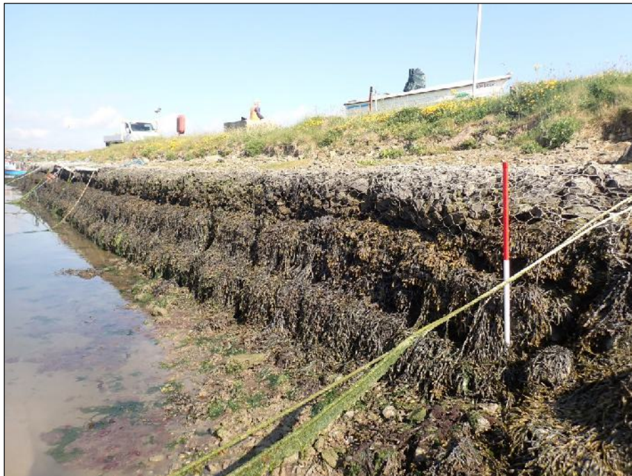
Plate 10: Northwest-facing view of stone filled gabions used to delineate the east side of the inner harbour area (1m scale).
