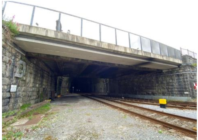
Figure 8-3 OBC405 N8 / Lower Glanmire Road Bridge is located between Kent Station and the Cork Tunnel
