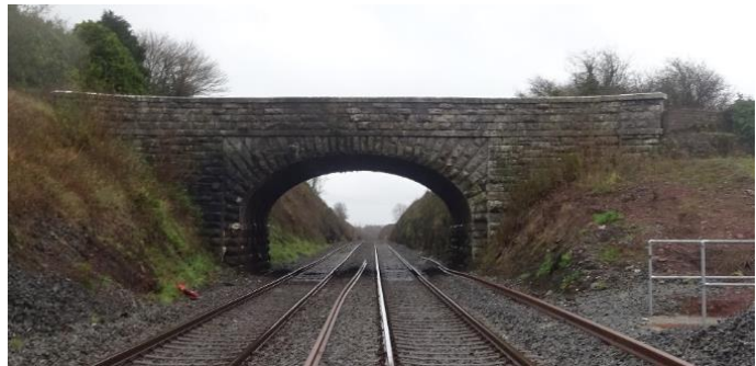
Figure 8-1 OBC394 Rathpeacon Overbridge currently has a clearance deficit of approx. 300mm
