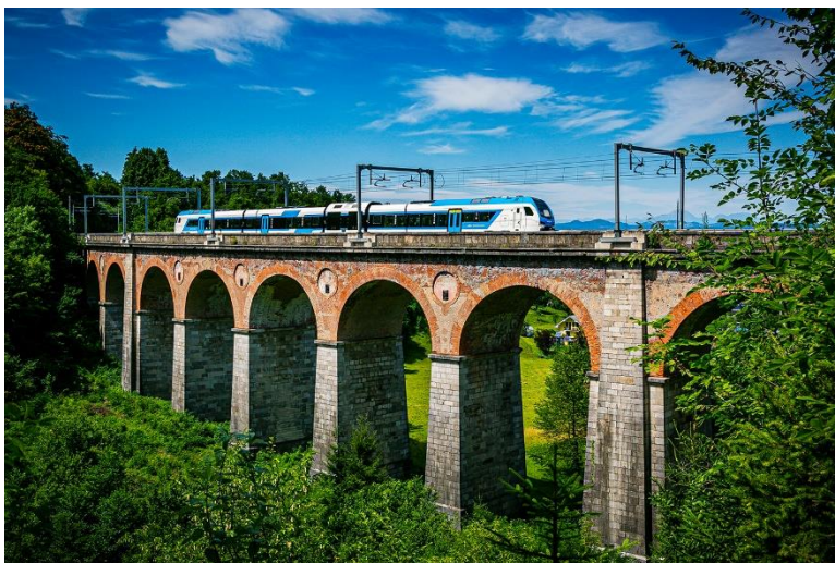
Figure 8-7 Photo of a typical OHLE system assembled on an existing stone railway bridge in Slovenia
